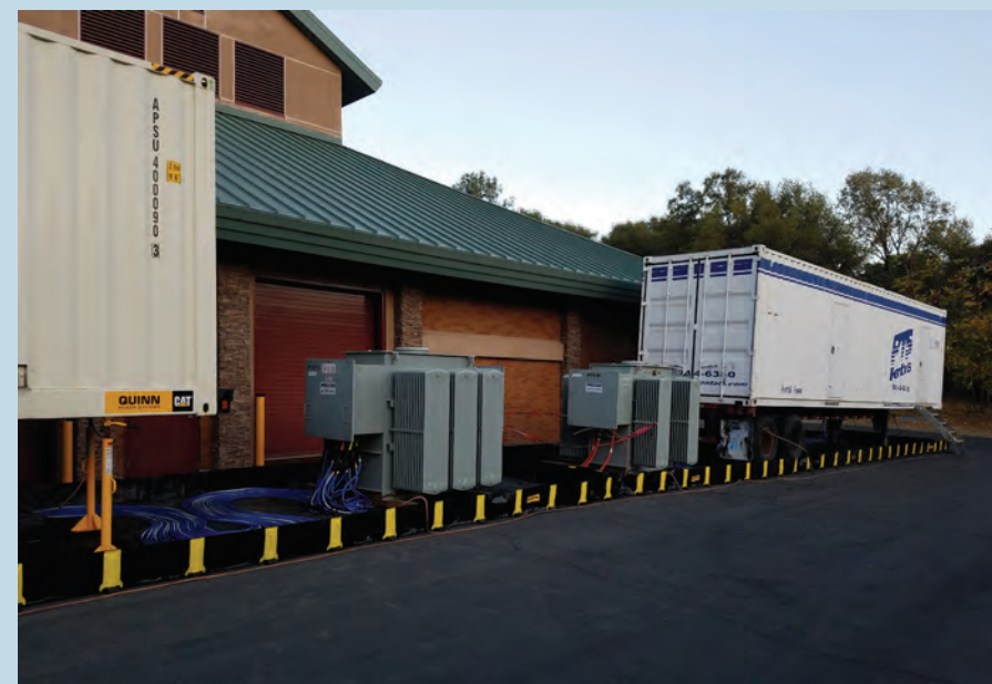
PG&E transported two 1.5-MW backup generators several hundred miles to Placer County, at no charge, enabling the water agency to continue pumping water during a PSPS in October. Photo courtesy of Placer County Water Agency
