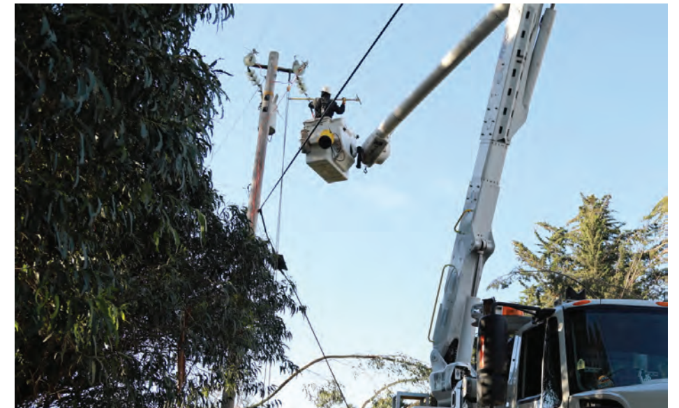
With wind speeds up to 88 mph and an elevated risk for a wildfire, SCE made the difficult decision to turn off power to some customers in Mammoth in mid-September.
