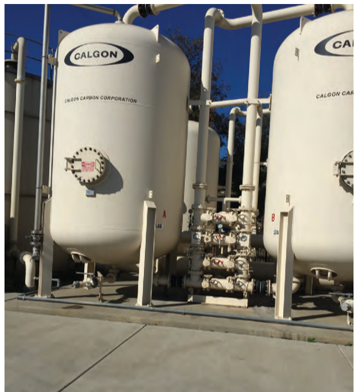
PFAS water-treatment vessels.
