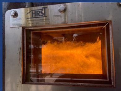
CoolVision™ Firing Duct Viewport
